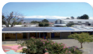
Solar Roof Costa Rica
