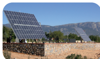
Solar Roof Mugla
